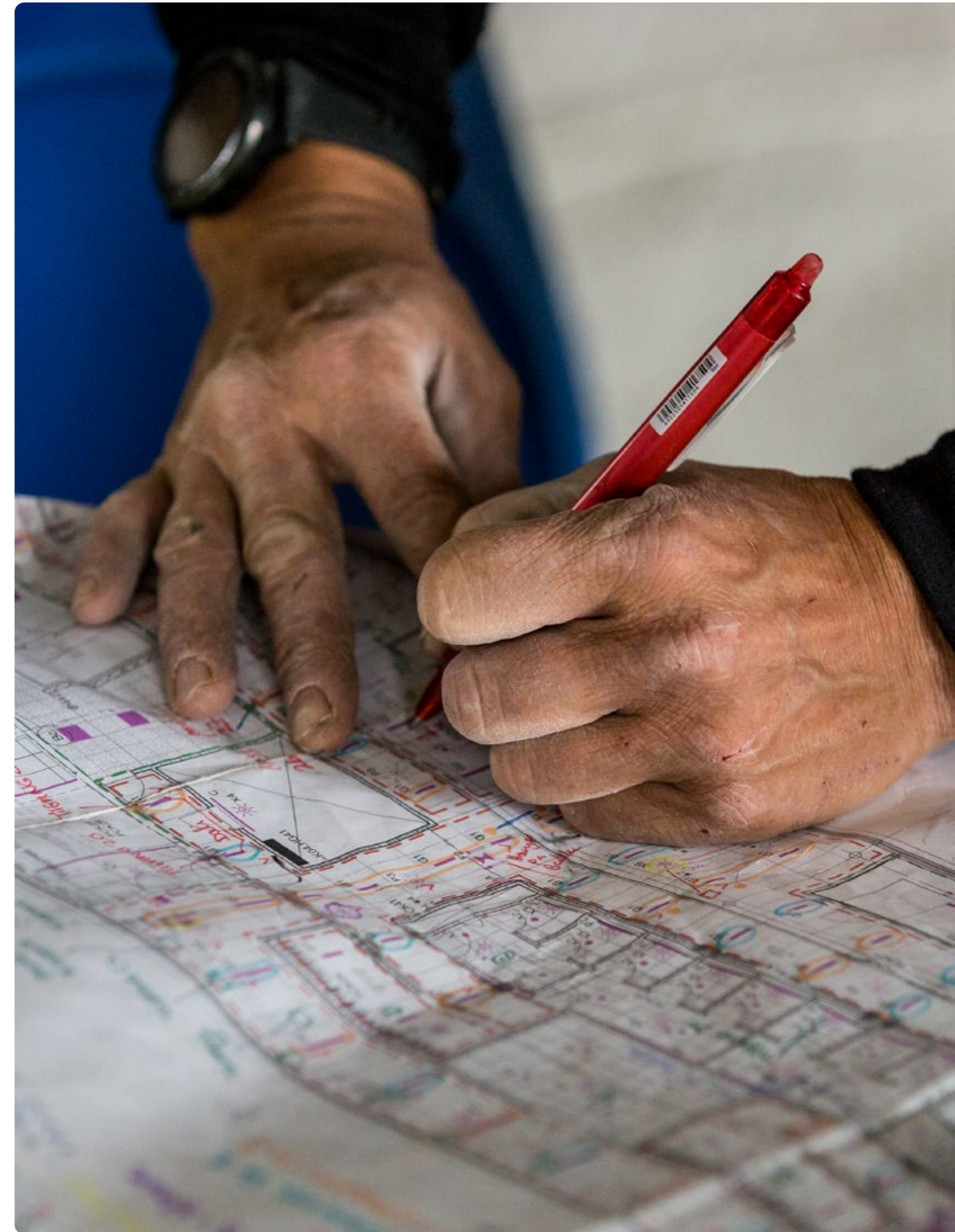
Jette, an electrician with NCC EL, working on DFDS' future domicile at Marmormolen, Copenhagen
